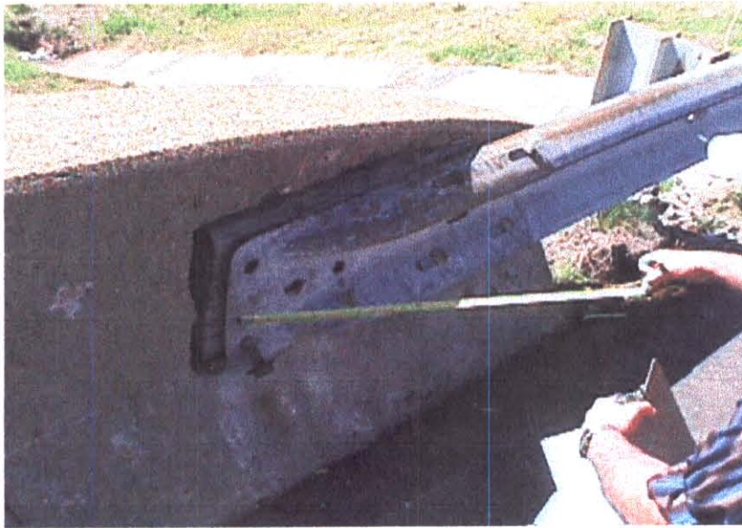
MISSING BOLTS IN TRASITION G RAIL
