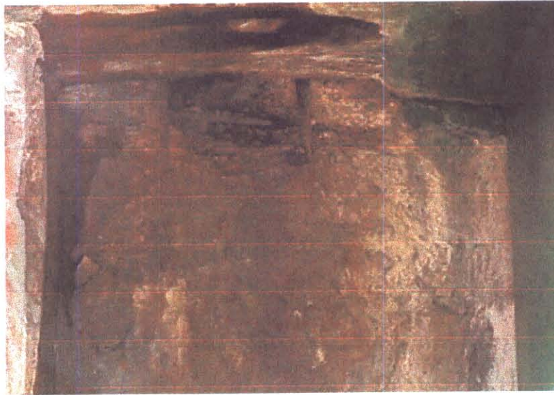
SPALL AT ABUTMENT #1 BACKWALL
