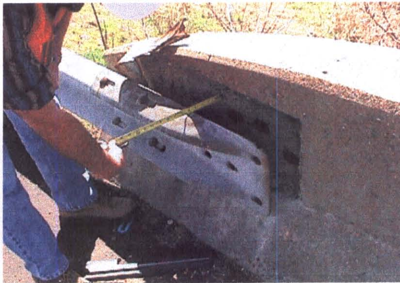
COLLISION DAMAGE GUARD RAIL TRANSITION RT. SIDE "B" END
