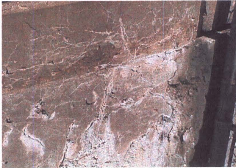
AREA OF DELAM TYPICAL ALL WINGS
