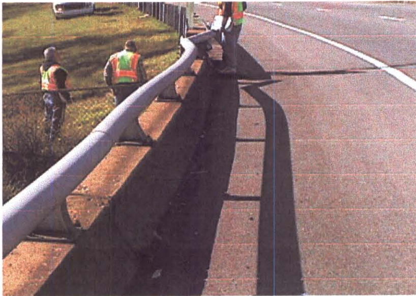
COLLISION DAMAGE AT SPAN #1 BRIDGE RAIL RIGHT
